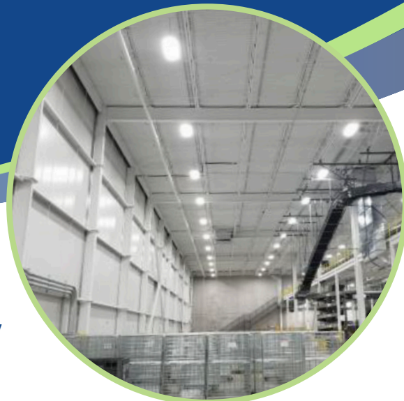
LED high bay fixtures with a networked lighting control system provided energy savings and enhanced lighting
