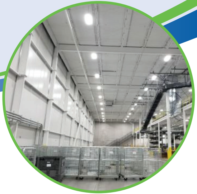
LED high bay fixtures with a networked lighting control system provided energy savings and enhanced lighting
